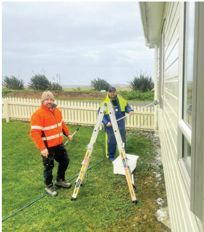
Tchiki Property and Vehicles, Duncan Ryan, helping to clean Kopinga's exterior walls with his brother and HMT trustee, Pana Ryan.
